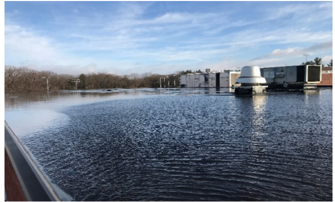
Dunmore Elementary School struggled for many years with malfunctioning roof drainage, shown above:
