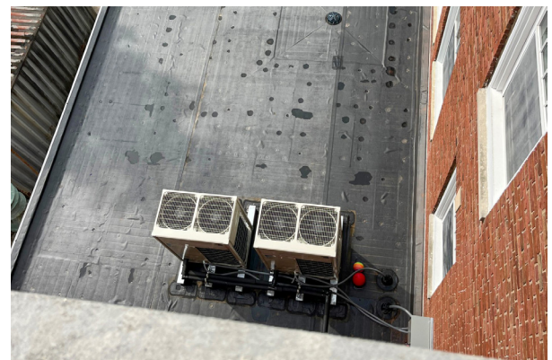
New Daikin variable speed rooftop units on roof
